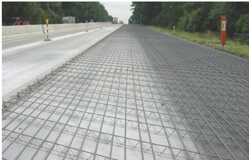
Figure 13: Image of the continuous reinforcement mesh for concrete pavement in CRCP (Source: BRRC)
